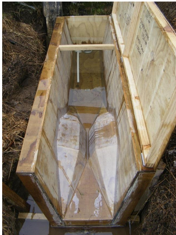
Figure 6: Waharoa farm (lower site) flume box. Pipe inflow (directed under culvert) can be seen in the upper part of the flume box.
