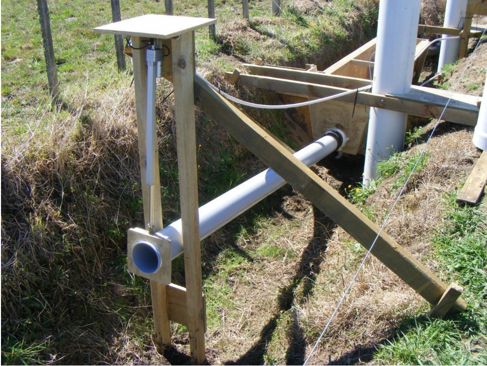
Figure 11: Tatuani farm (upper site) drain water intake pipe and flume box. Photograph is taken looking downstream.
