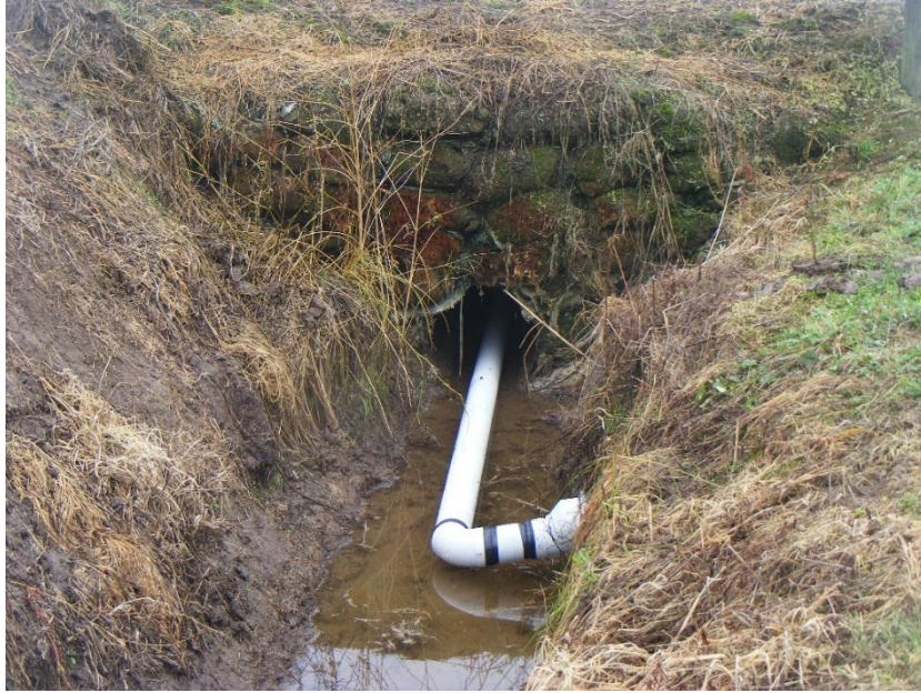
Figure 5: Waharoa farm (lower site) drain water collection pipe connected to the 160 mm subsurface pipe. Water flows from out of the 160 mm subsurface pipe (which collects water from a series of 110 mm perforated subsurface drainage pipes). Because of the position of a culvert at this site water is piped to the flume box on the other side of the culvert.
