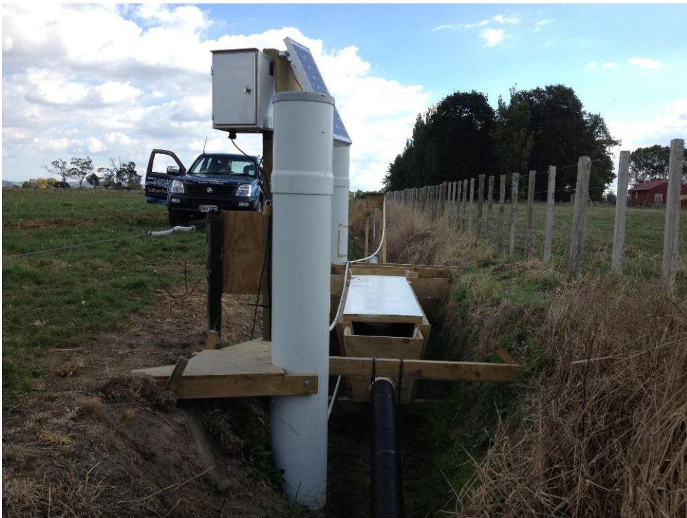
Figure 12: Tatuani farm (upper site) flume box and stilling wells. Photograph was taken looking upstream. All flow from the flume box discharges into a 150 mm pipe (black pipe) and is diverted past the lower flume site.
