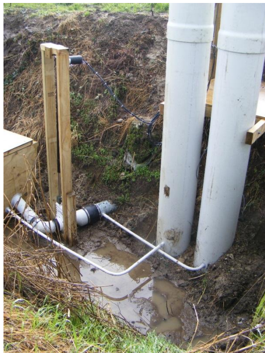
Figure 8: Waharoa farm (upper site) subsurface drain water diversion setup. Photograph shows diversion of 160 mm subsurface drain into flume box. Wooden structure located on either side of the diversion pipe is the gate valve unit that controls level of groundwater in the experimental area.
