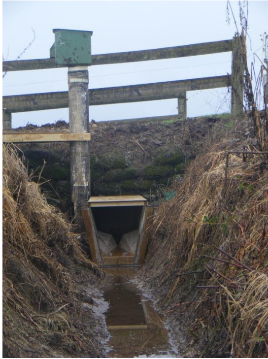
Figure 7: Waharoa farm (lower site) flume box and stilling well. Photograph was taken looking upstream.
