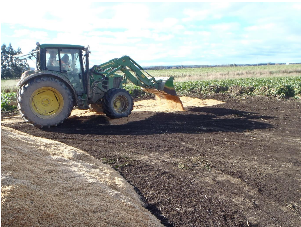
Plate 1: Sawdust being laid over a lignite base to form a temporary stand-off pad.
