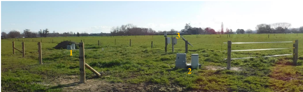
Figure 2 Photo of the completed installation of the woodchip bioreactor showing the main components: (1) inlet control structure with auto sampler and stilling well, (2) outlet control structure with auto sampler and stilling well, (3) rain gauge, solar panel, and control panels for the instruments.
